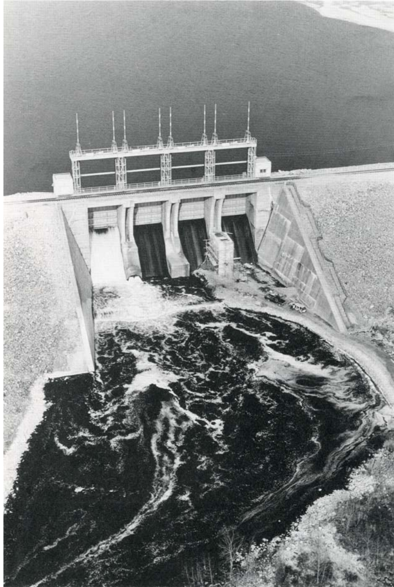
Close-up of the Shand Dam during construction of the hydro generating unit. Water is being released from one of the main gates, as well as the left 48" low flow discharge tube. The main 60" discharge tube in the middle of the spillway is closed, while the hydro generating station is being constructed over the right 48" discharge tube.
