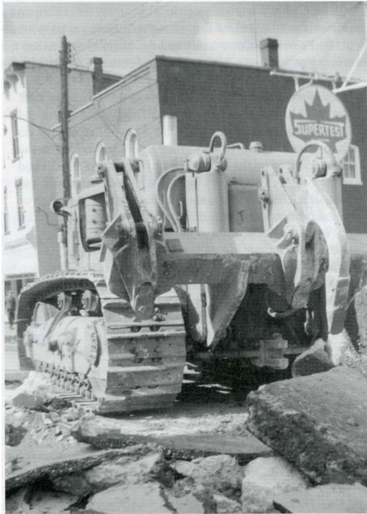
Installation of sanitary sewers, George and Smith Street, Village of Arthur, 1960s. FROM THE COLLECTION OF THE WELLINGTON COUNTY MUSEUM AND ARCHIVES, PH 14501.
