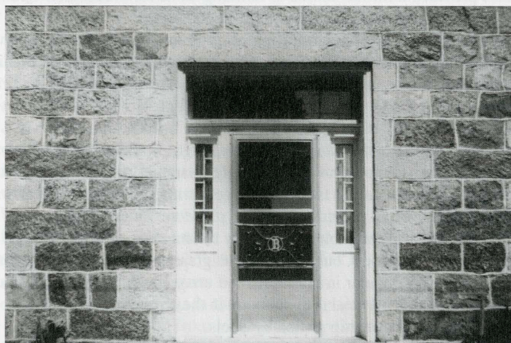
Ashlar coursed masonry with continuous horizontal levels. The lighter blocks (quoins) which frame the openings are of dressed limestone, while the darker background masonry is of split field granite. Laidlaw-Bender farm, Lot 12, Concession 3 B, Guelph Township.
