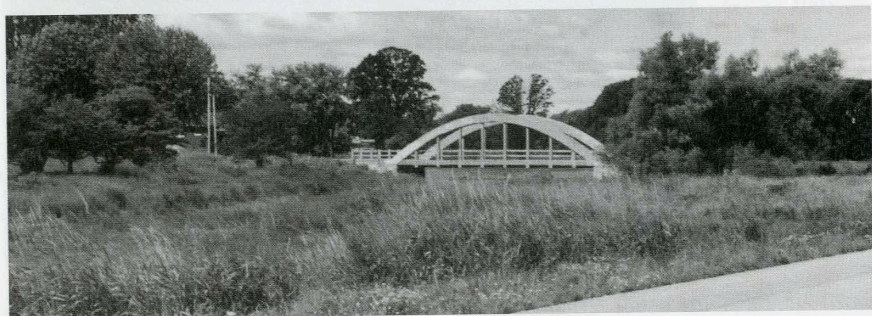
Concrete bowstring bridge, erected ca.1915, near the cheese factory, Concession 13, Maryborough Twp.
